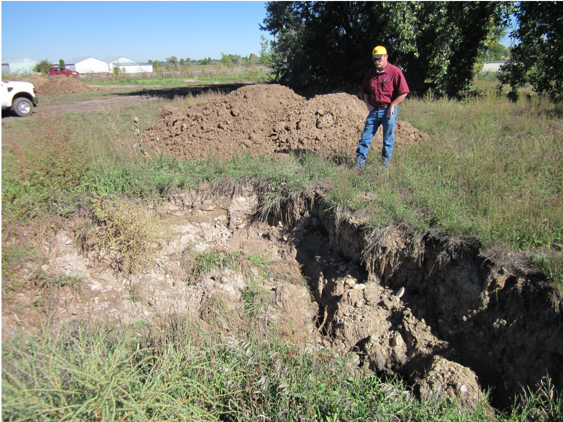
Irrigation damage as a result of the 2013 flood. Recovered soil went to companies to repair flood damage.
